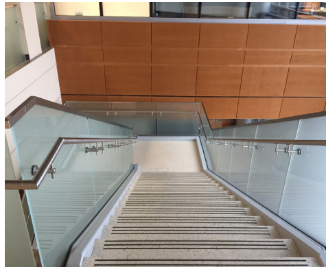
The addition of a stainless top cap added glass edge protection and rigidity
